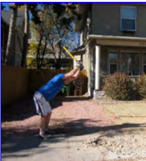
Adam Brink works to demolish an old section of sidewalk, so that ONEN sponsor Groninger Concrete can pour new concrete. (Fall, 2010)
