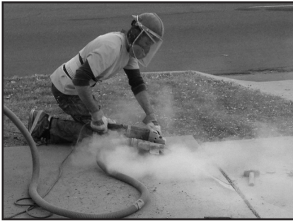
An employee from Precision Concrete Cutting demonstrates sidewalk shaving at 1335 N. Weber in November 2012.
